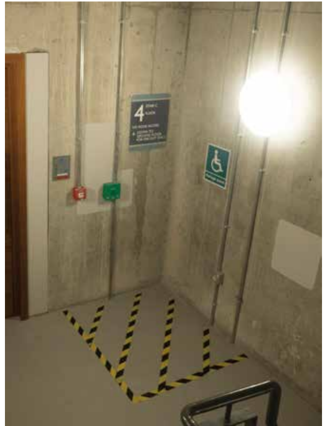
Figure 14 Ensure disabled peoples' refuges on landings and their intercoms are directly lit
