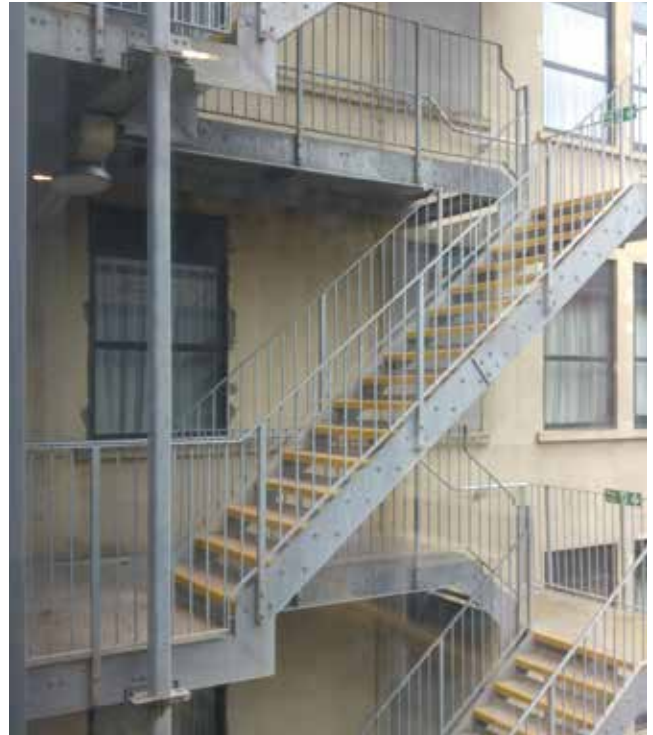
Figure 26 Emergency lighting and signage are needed on rarely used external escape routes, which may be wet or covered in snow/ice
