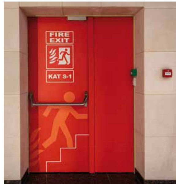
Figure 16 Directly light final escape doors to ensure escapees can operate any opening mechanism or unusual security release buttons (© Mehmet Cetin/Shutterstock)
