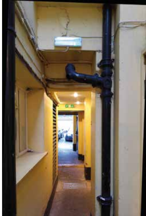
Figure 22 External exit signs may be needed for alleyways and divided routes leading towards place of safety
