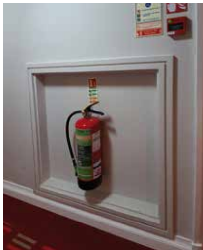
Figure 5 Ensure all fire-fighting equipment and break-glass call points are directly lit
