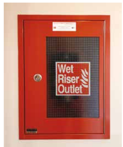
Figure 6 Ensure dry and wet risers are directly lit
