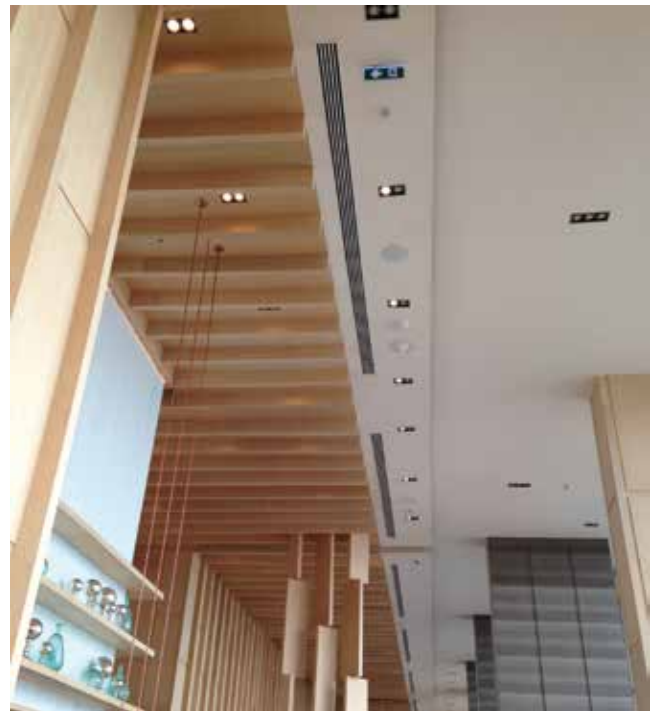
Figure 20 Ensure that exit signs are roughly along normal lines of sight and not installed too high above normal eye-line. In an emergency would you have seen the exit sign in this image?
