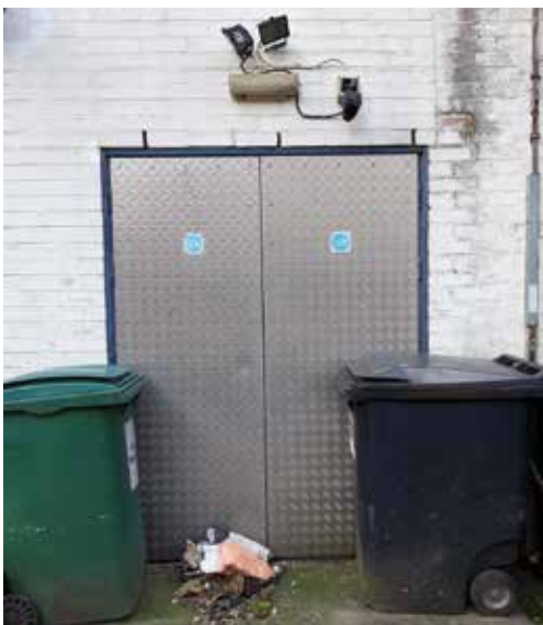
Figure 23 Light areas outside of final exit doors to assist escapees in moving any external obstructions and to assist them move away from the doorway quickly and safely
